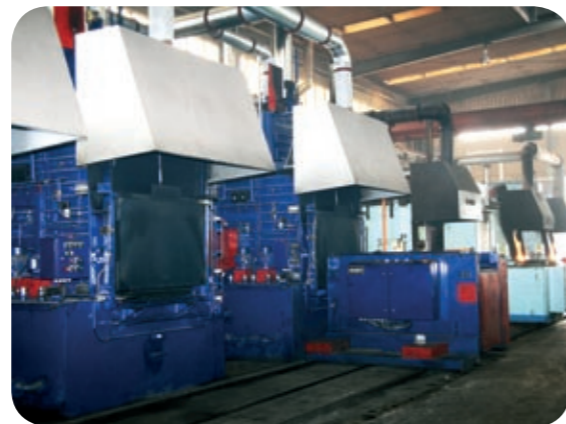
Furnaces for heat treatment process
